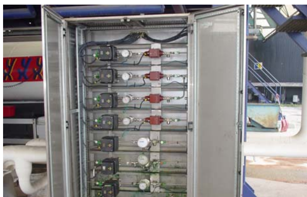
Picture 2: Cabinet with multiple injectors
